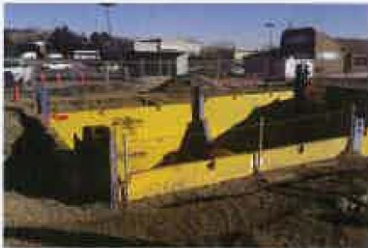
An NTS engineered slide rail system shored the launch shaft for an under-road storm sewer in Colorado.
